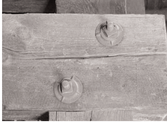
Fig. 4. Split between bolts caused by wood shrinkage.
