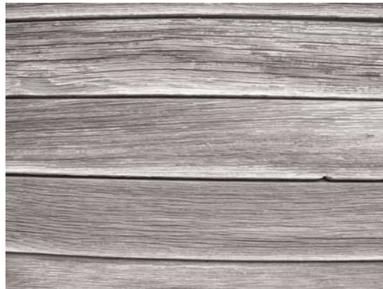
Fig. 5. Weathered cladding, considered aesthetically pleasing.
