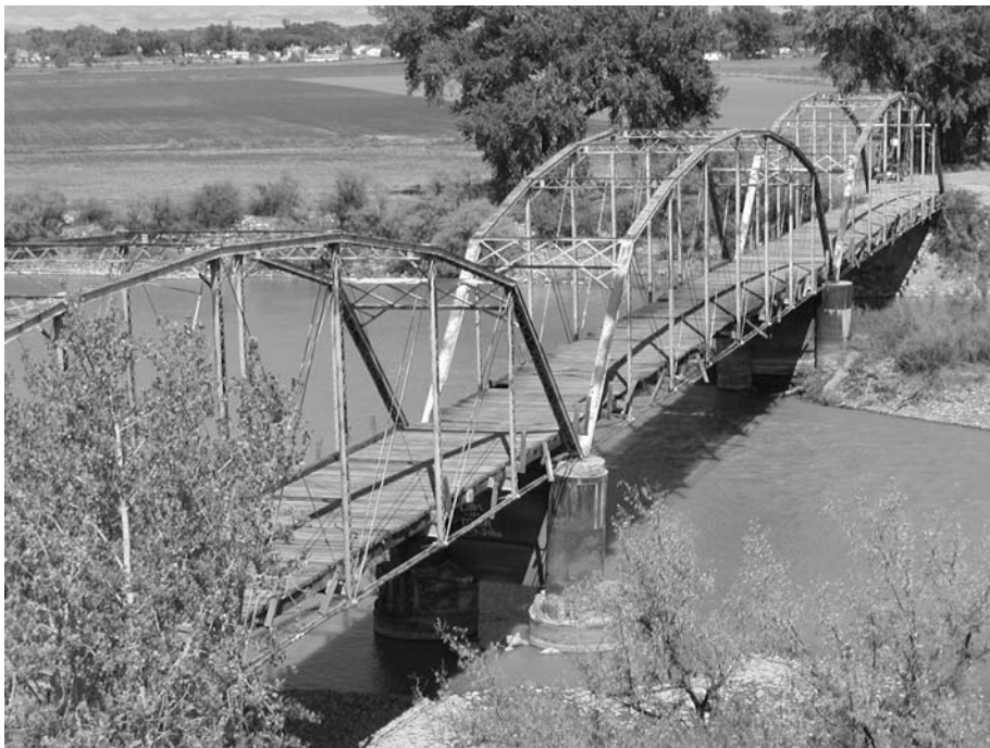
Fig. 1. Fruita Bridge over the Colorado River, near Fruita, Colorado. This Parker truss, built in 1907, has three 155-foot (47-meter) spans, each with eight bays. Its deck consists of timber deck planks spiked to timber stringers, which bear on steel floor beams. The deck is discontinuous, with gaps between the deck planks. All images by the authors.
