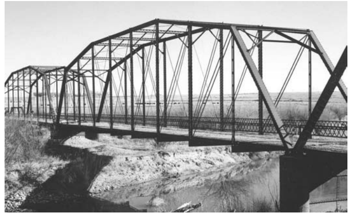
Fig. 3. Prowers Bridge over the Arkansas River, near Lamar, Colorado. The span selected for study is a nine-bay camelback Pratt through truss of 160-foot (49-meter) span, built in 1909. It has steel floor beams with steel stringers, covered by a corrugated-metal deck with asphalt pavement.
