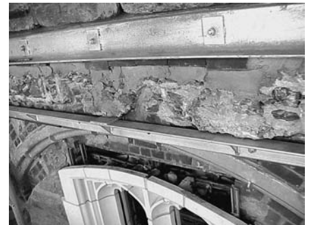
Fig. 5. Galvanized-steel supports for resin-based, thin-shell units replacing original terra cotta at Shepard Hall. Courtesy of Robert Silman Associates.
