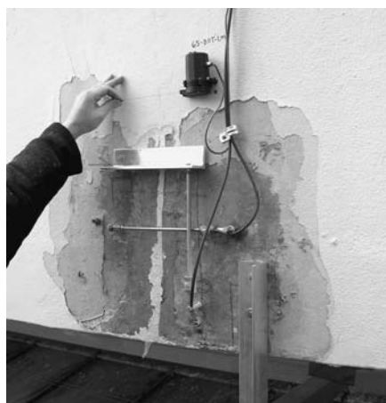
Fig. 3. Crack monitor installed at the Guggenheim Museum. Courtesy of Robert Silman Associates.
