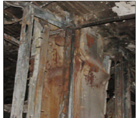
Failure of the fireproofing allowed this built-up column to buckle at the eighth floor of a 25-storey, early twentieth century building. (Photo: Derek Trelstad, LZA Technology)
