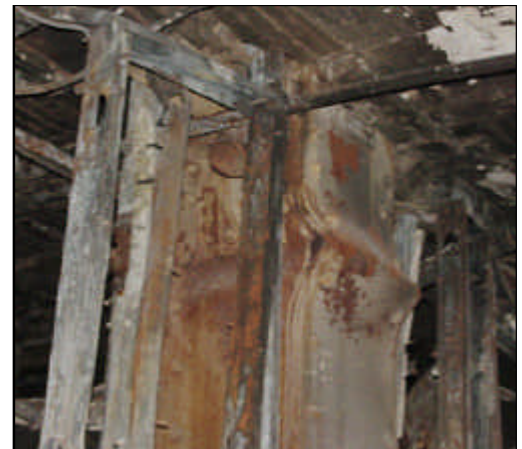
Failure of the fireproofing allowed this built-up column to buckle at the eighth floor of a 25-storey, early twentieth century building. (Photo: Derek Trelstad, LZA Technology)
