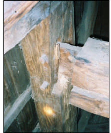
Damage to the wood girt, caused by an insect infestation, resulted in failure of the mortise-and-tenon connection in this late eighteenth century church building. (Photo: Derek Trelstad, LZA Technology)
