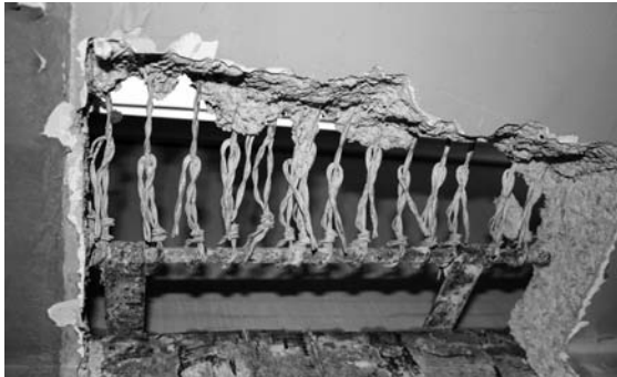
Fig. 5. Probe at the inside face of a spandrel beam showing wrapped attachment of the wires to secondary steel.
