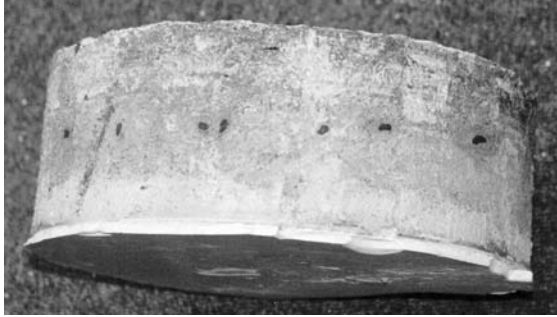
Fig. 4. Core through floor showing the thin layer of finish plaster on bottom and the cut ends of wires.
