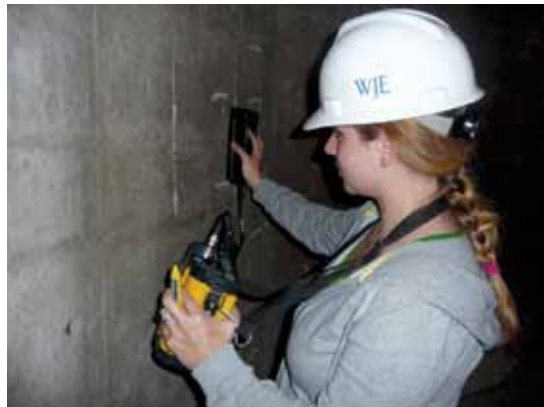
Fig. 10. Use of nondestructive testing to determine location of reinforcement steel during an assessment of a concrete structure.
