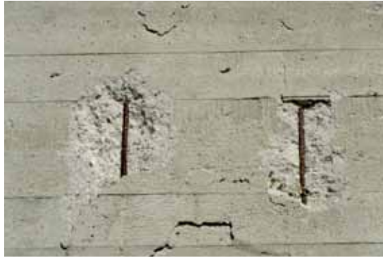
Fig. 8. Delamination and spalling in exposed concrete, documented as part of the visual condition survey. Photograph by Adrienne Goetz, WJE.
